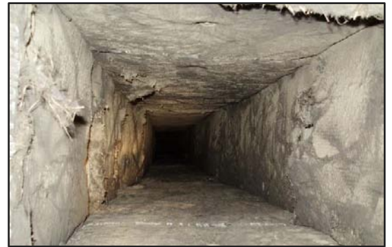
Microbial growth on internal duct liner
