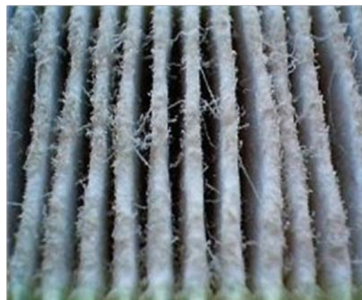
Contaminants trapped in HEPA filter.
