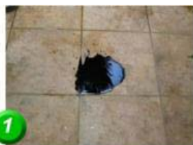
1 Dirty motor oil on the floor.
