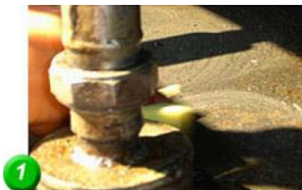
Stainless steel tank contaminated with filler and thick lubricant oil for years.
